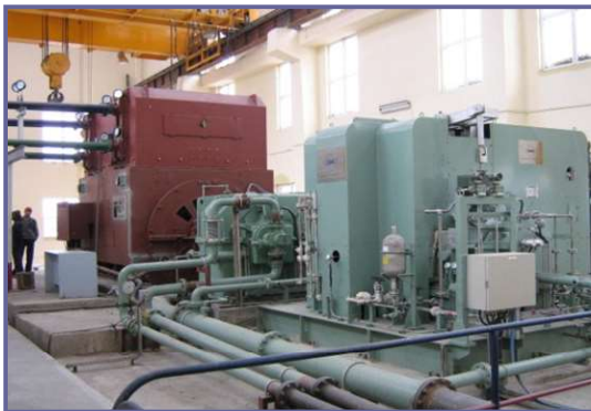
Vibration measurements and on-site balancing of 25 MW turbine-generator assemblies at a sugar mill
