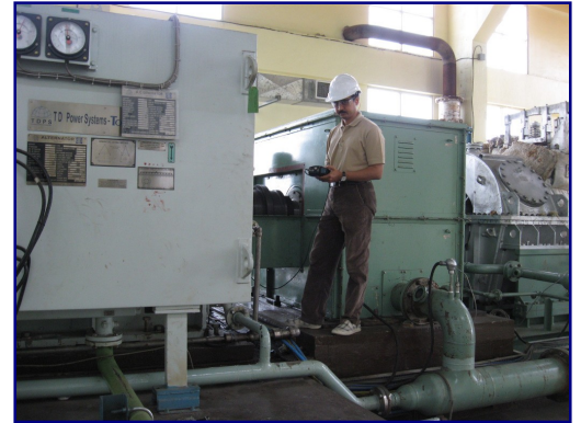
Vibration studies on 12.5 MW generator assembly at a paper mill in Philippines
