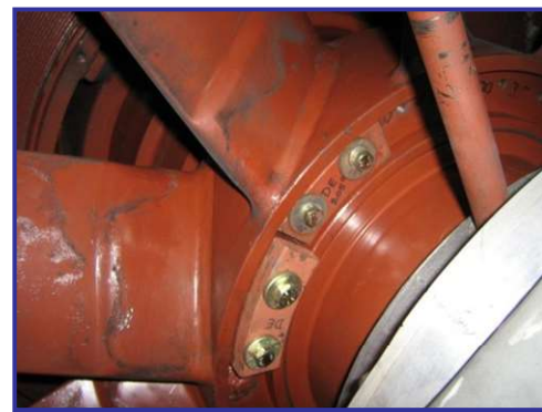
One of the corrections mass added on the 25 MW generator fan assembly during on-site balancing
