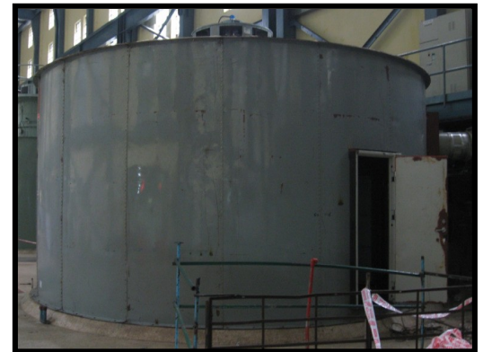
Vibration studies and on-site balancing of 60 MW hydro generator (112 tons) at Sabarigiri hydro power station,
